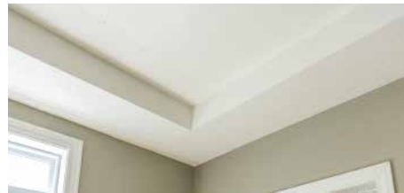
Tray Ceiling with 4 recessed can lights OP19011AR
